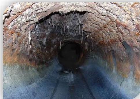
Corrosion due to gas attack
