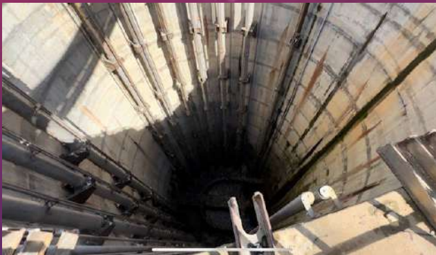
Nancy Creek Tunnel Pump Station – Discharge Pipes to Treatment Facility
